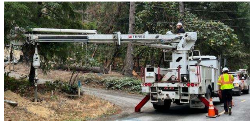
California Advanced Services Fund Infrastructure Project: Hunter's Hoopa Valley Broadband Initiative to serve 1,198 households of the Hoopa Tribe in Humboldt County. Pole placement using an auger to drill hole for pole placement.
