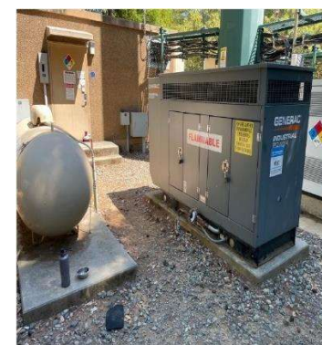
Macro cell site fixed generator, Myers Flat, Humboldt County
